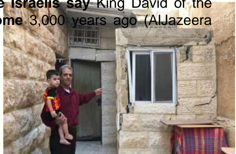
Picture 7: Fayyad Abu Rmeleh shows the cracks and deformations that have formed in his home from Israeli excavations [Dareen Jubeh/Al Ja
